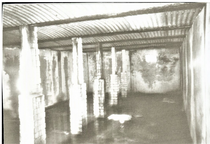
The underground tank at West End (Syd Flatman)
